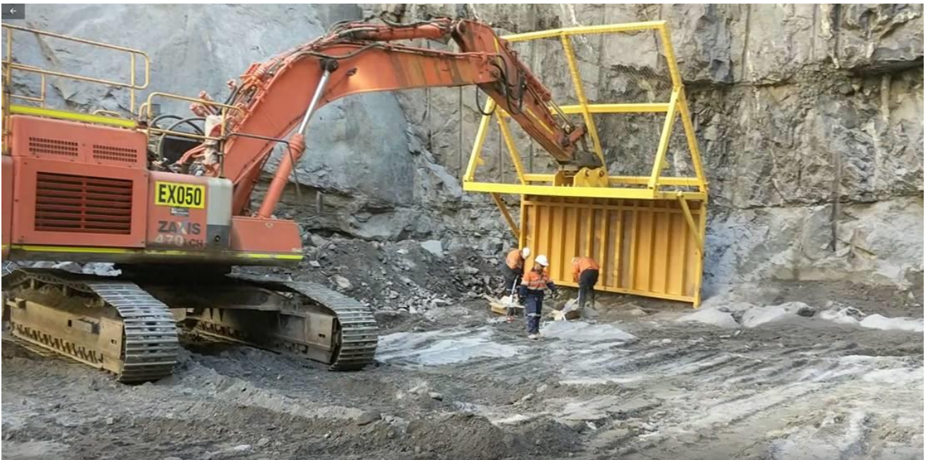
FIGURE 3. ROCK FALL SHELTER
