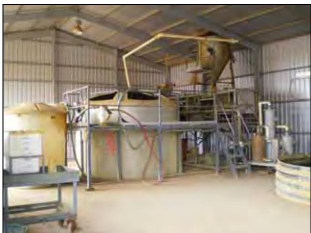
Copper oxide processing plant
