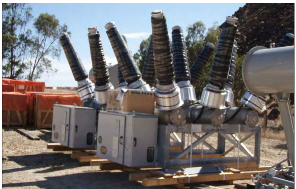
High Voltage Switchgear
